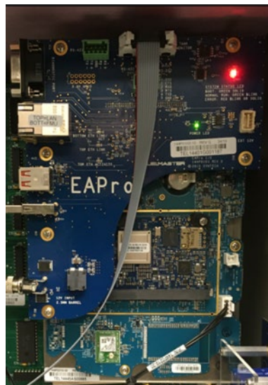
Figure 26 TMU Cable Connected to EAPro
