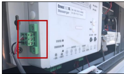
CrossTalk Controller showing 3-pin Connector Installed
